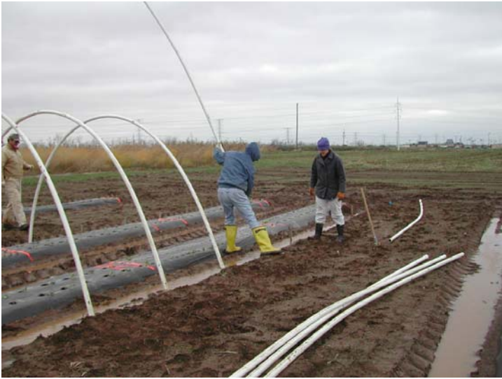
Figure 4. Placing the PVC pipes over the anchors and bending them to the adjacent side
